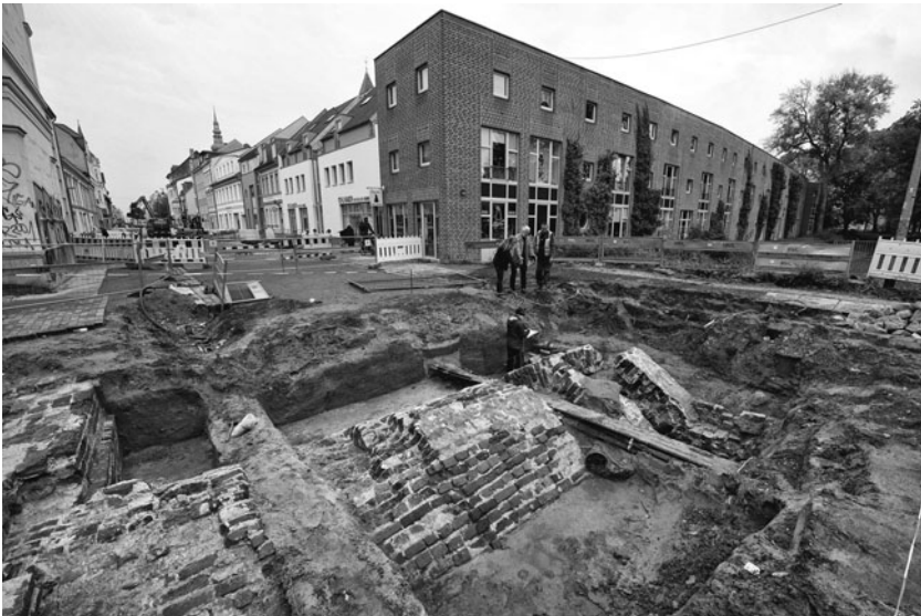
Figure 14.1 A medieval vaulted tunnel dating to about A.D. 1300 unearthed during road construction work in Greifswald, Germany, October, 2014.
